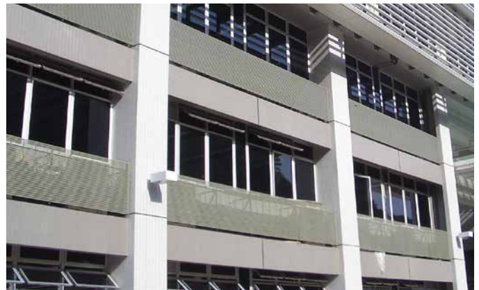
Strongwell DURADEK® I-6000 grating was installed at this School of Business and Information Systems in Hong Kong as air-conditioning platforms when placed horizontally and as louver when placed vertically (as shown here).
