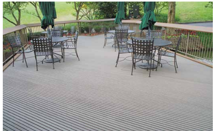
The Muirfield Village Golf Club, designed by Jack Nicklaus, offers an outside patio deck for players to relax and have a snack between nines. After years of constant moisture and the steady pounding of golf shoes, the wood deck had become a safety hazard and required replacement. Strongwell manufactured DURAGRID® T-1800 using a custom pigmented resin to replace the wooden deck to offer both the aesthetic and structural benefits the club was looking for.
