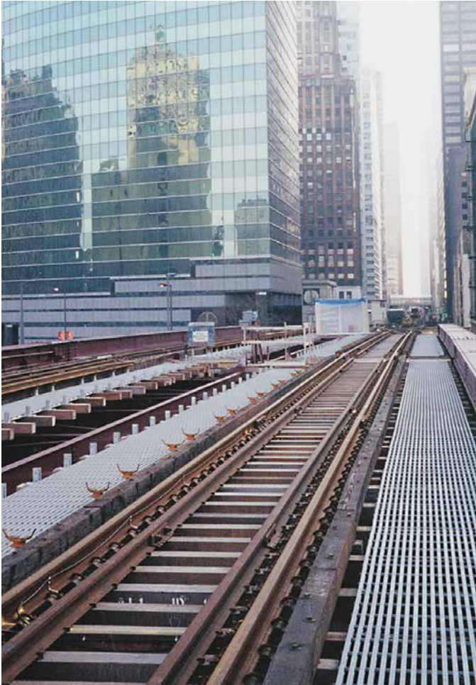
Chicago Transit maintenance walkways alongside elevated train tracks constitute one of the largest fiberglass grating installations in history. This project used DURAGRID® T-5000 2" with a custom polyester resin.
