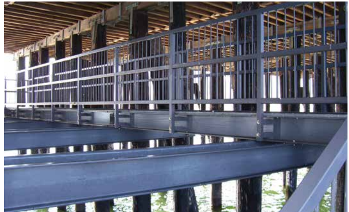
The Avila Beach Pier in California was reconstructed using EXTREN® structural shapes for support, DURADEK® pultruded grating, stair treads and handrail.
