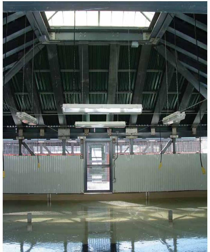
The Craig Brook National Fish Hatchery in East Orland, Maine used corrosion resistant EXTREN® structural shapes to frame roofing structures over moisture rich crowding pools.
