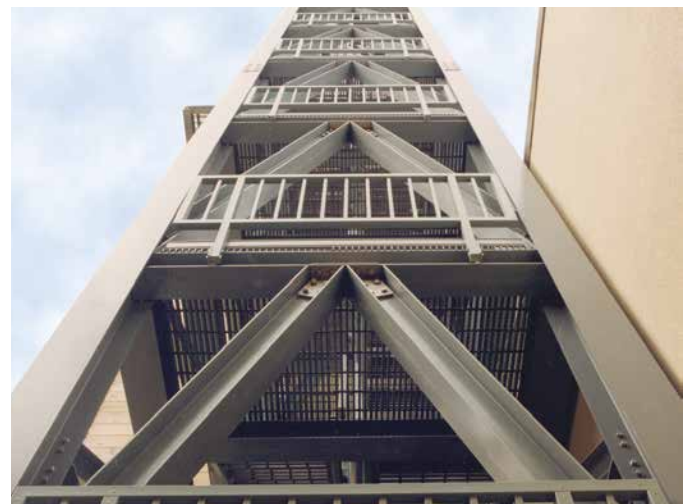
A 63' (19.2m) high freestanding fiberglass stair tower at Ft. Story Army Base, Virginia Beach, Virginia.
