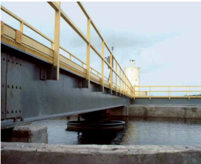
Lightweight, corrosion resistant 24" (610mm) I-beams span 45' (13.7m) to bridge clarifiers at the Las Rusias, Texas wastewater treatment plant.
